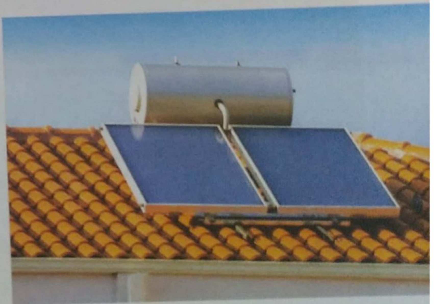
Solar Water Heater
