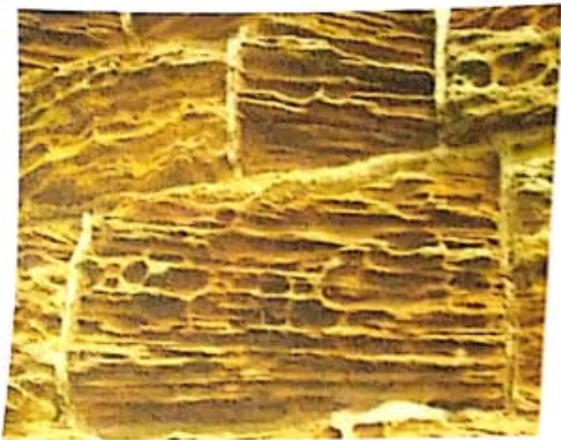
Chemical Weathering of Sandstone
